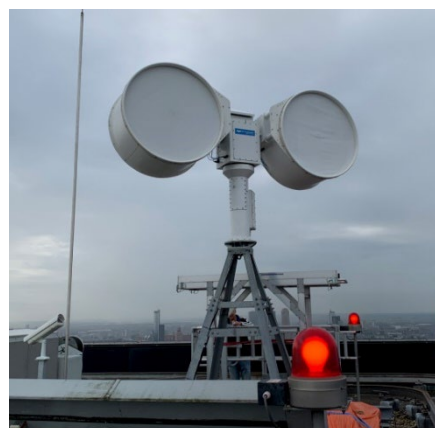
Fig. 1 X-band Radar Rijnmond deployed and operated in Rotterdam
